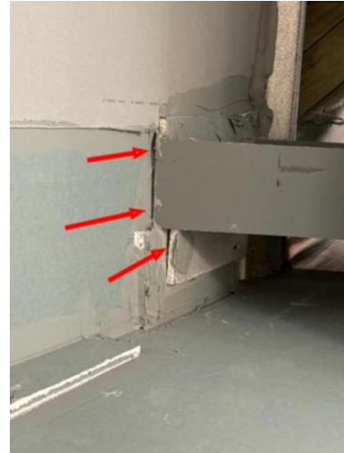
Figure 4. Smoke wall not continuously sealed
