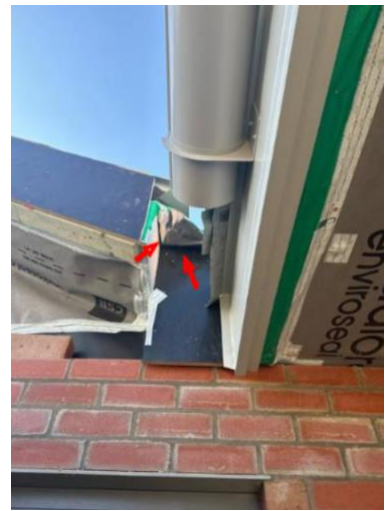
Figure 6. Seal at roof/wall junction not continuously sealed
