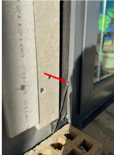
Figure 3. Cable penetration not sealed
