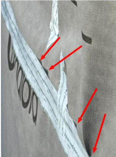
Figure 2. Air barrier membrane not taped correctly
